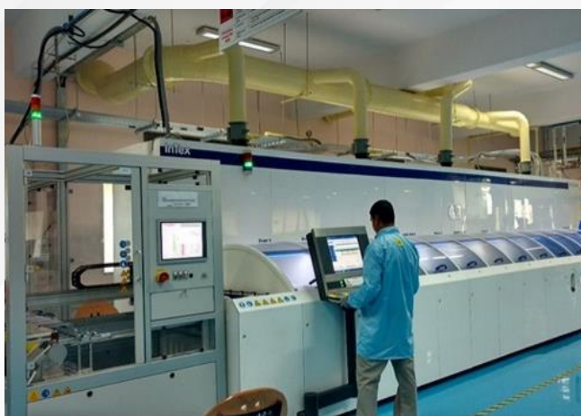
Acid Texturing Station of Solar Cell Manufacturing Facility
